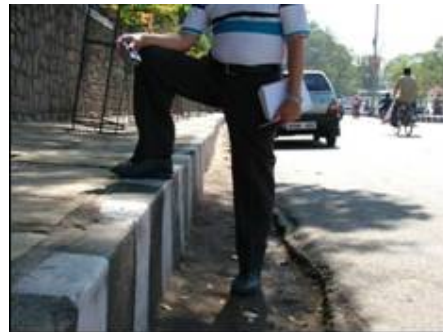
Curbs over 18 cm are very inconvenient for pedestrians.
