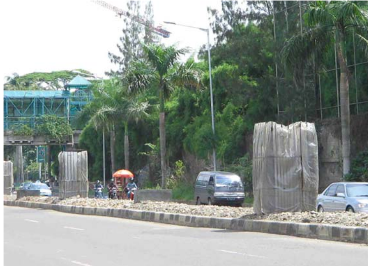
Ten months after monorail construction was officially inaugurated in Jakarta in June 2004, the project has foundered due to the private developer's demands to the city for additional funding.
