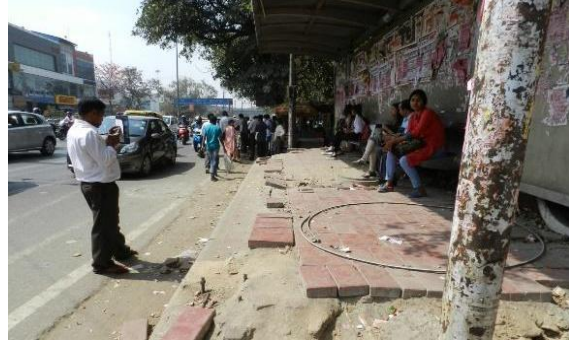
Image 5: Broken footpath at Kirti Nagar bus shelter
