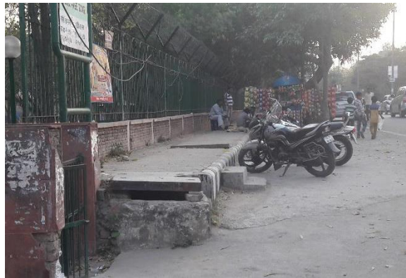
Image 21: Inaccessible footpath height
