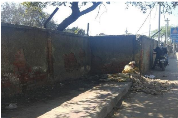
Image 8: Discontinuous footpath near Ambedkar Nagar bus terminal
