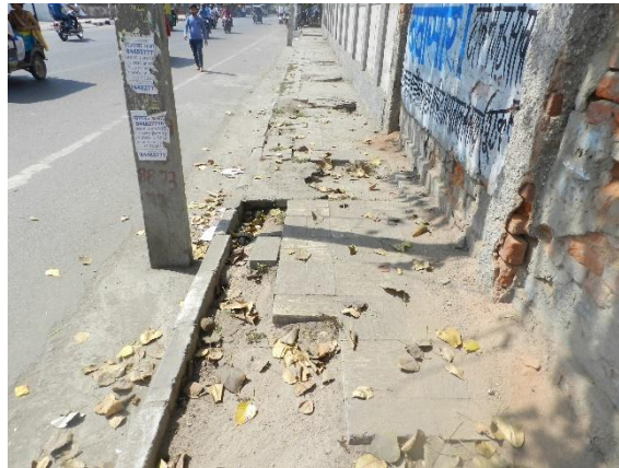
Image 22: Poor footpath surface
