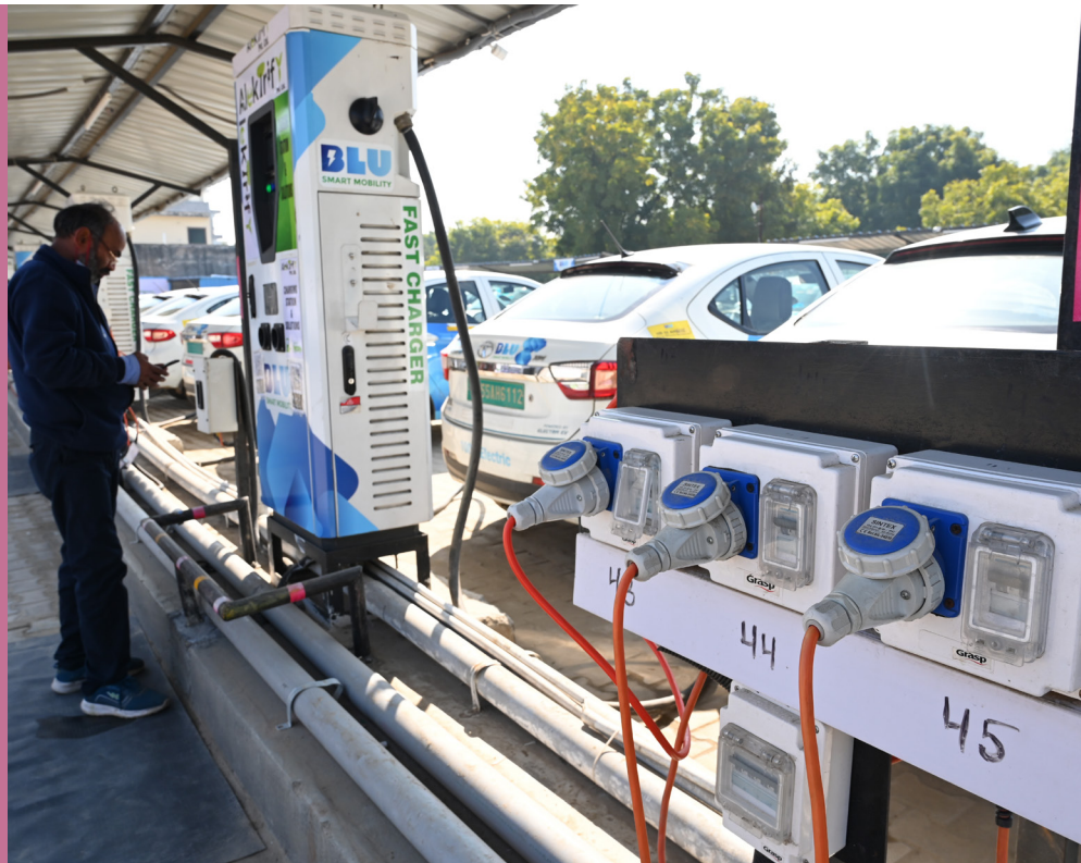
India's largest EV charging station in Gurugram, the business capital of Haryana. SOURCE: Sudarshan Jha via Shutterstock
